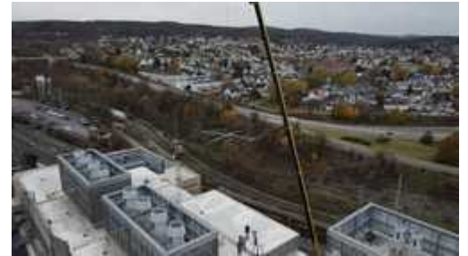
A crane lifts an antenna into place for W3USR's new location. [Photo courtesy of Byron Maldonado, University of Scranton]
